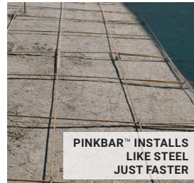
CORRODED #4 STEEL REBAR FROM 5-YEAR-OLD 6" THICK CONCRETE PAD THAT WAS REPLACED WITH PINKBAR™
